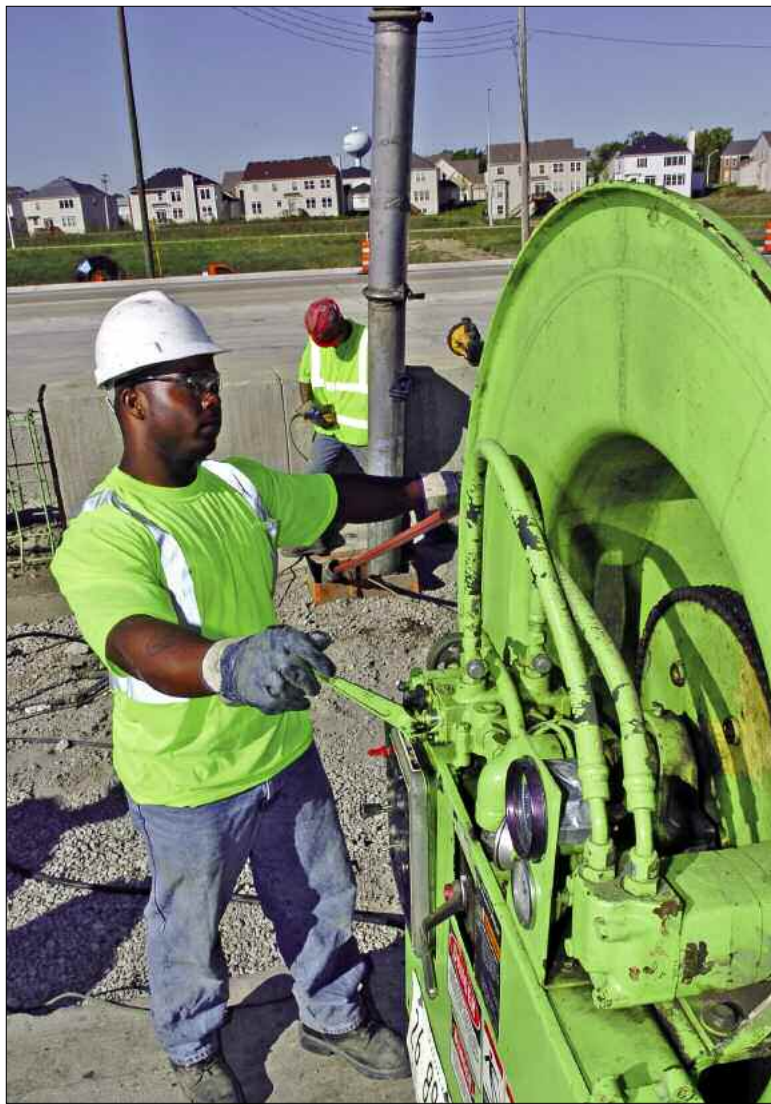
Larry Jeffries operates the jetter on a combination unit as Chuck Cushing vacuums debris.
