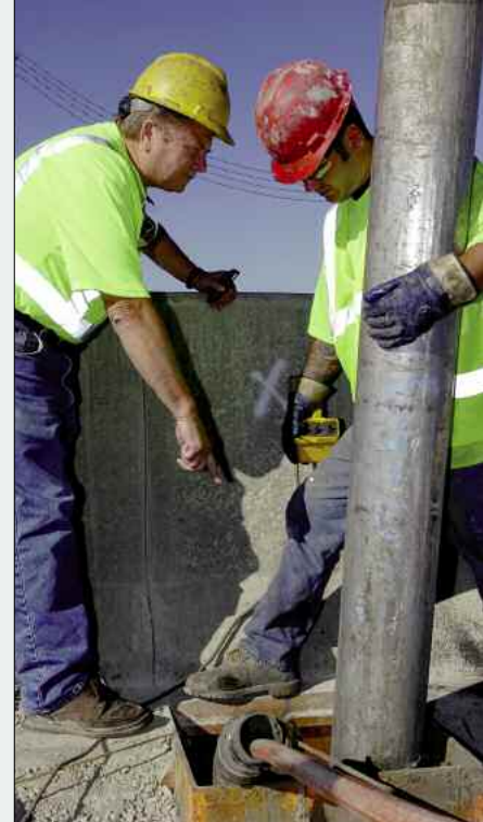
Owner Al Kulig (left) and operator Chuck Cushing discuss progress on an obstructed sewer line.
